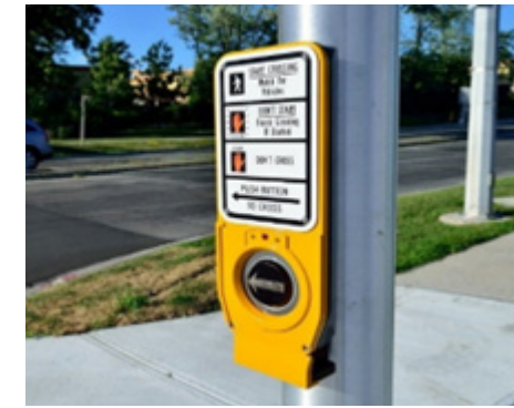
Accessible Pedestrian Signal (APS)
